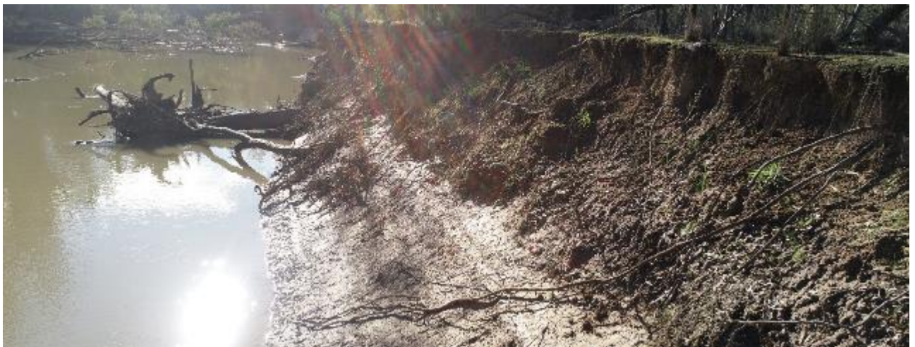
Figure 9.37 Drone photograph taken on the final visit (visit 4: 14/07/2020) highlighting areas of the bank that appear to have experienced mass-failure events within the monitoring period. Edward/Kolety River downstream of Stevens Weir.
