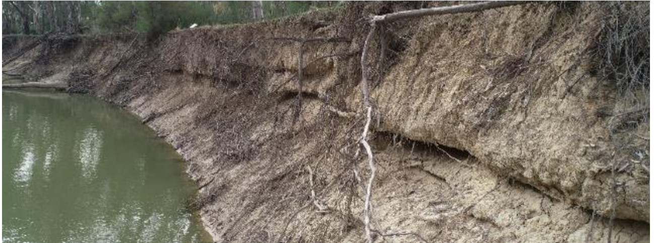
Figure 9.36 Drone photograph taken on the 3 rd visit (07/04/2020) highlighting the notch at the site in the Edward/Kolety River downstream of Stevens Weir
